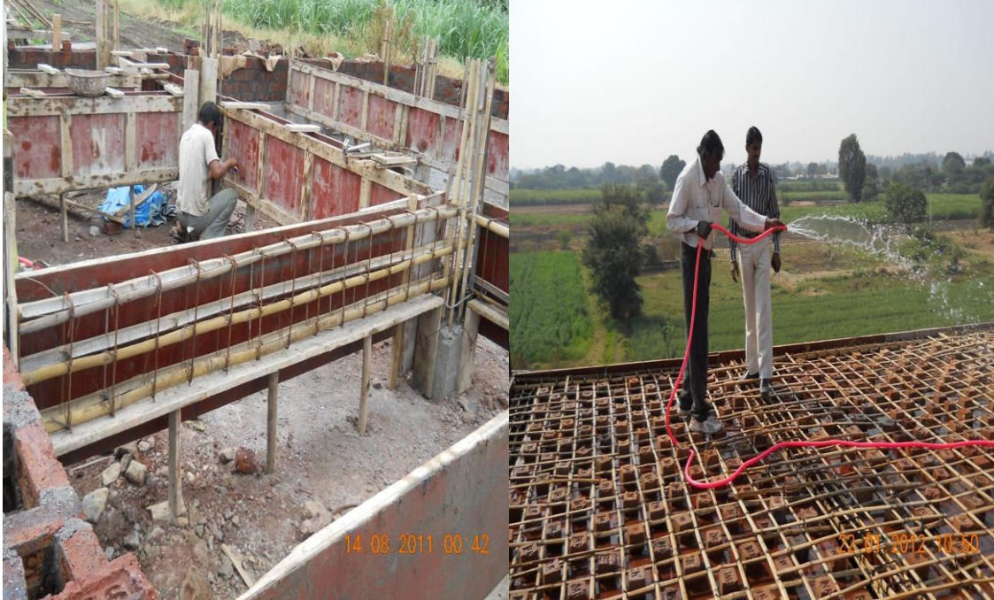
Figure 2.3: Bamboo as replacement for steel in slab, beam and column construction (Online Image)
