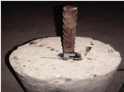
Figure 9a: Pull through failure mode
