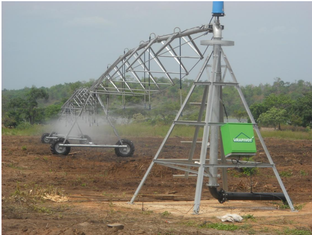
Figure 6. The 20 ha (4 -span) Center pivot system installed at Ikere Gorge dam.
